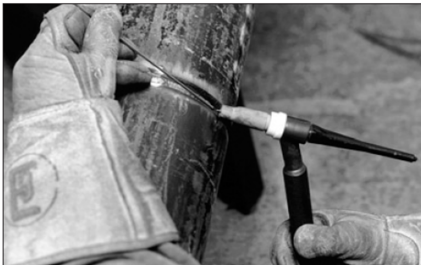
Figure 8.13 Demonstration of how the torch and filler rod are held to accomplish the "walking-the-cup" method of pipe welding.
