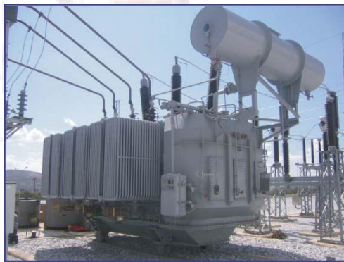
Transformer 150/20KV 50MVA
