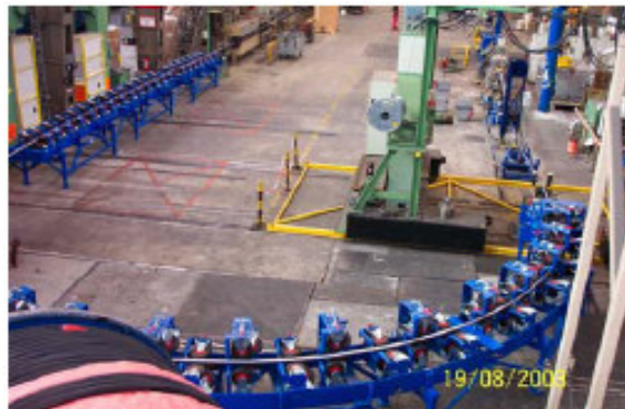
Photo 2: 180° loop between lead extruder (right) and outer sheath line (left)
